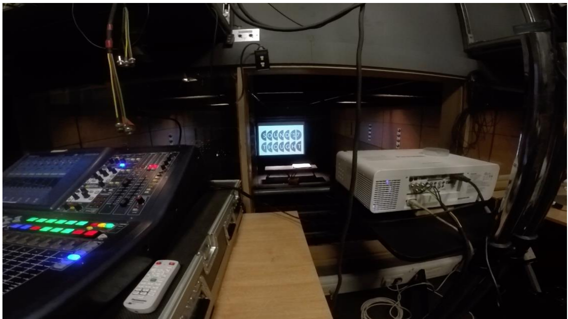
Sound Thought control room.
